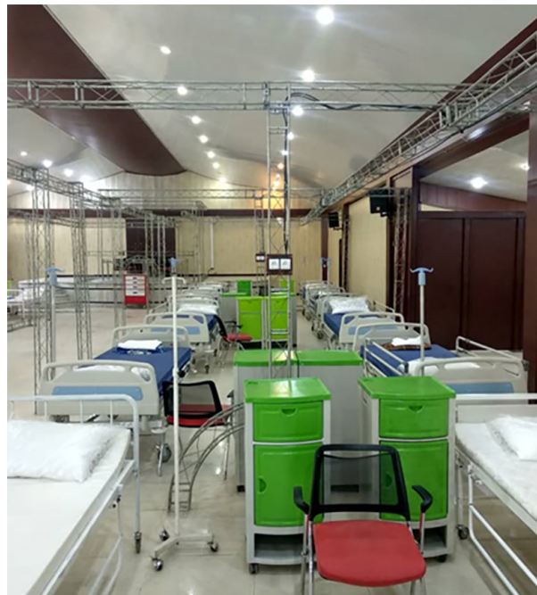
Figure 1. Photograph of the COVID-19 Police Field Hospital in the final stages of construction.
