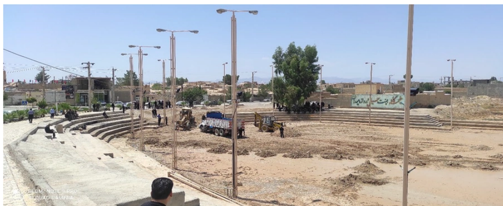
Figure 2. Drainage operations using fire department equipment and community volunteers.
